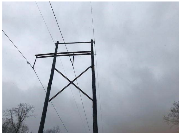
The stress related cross arm break on structure number 36 at Belleville
